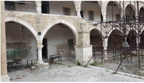
Figure 8 – The scaffolding is holding in place the leaning column, urgent intervention is required (photo: A. Camiz, 2014).
