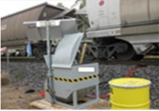
Figure 4. Solar operated electrical lubricators [19]
