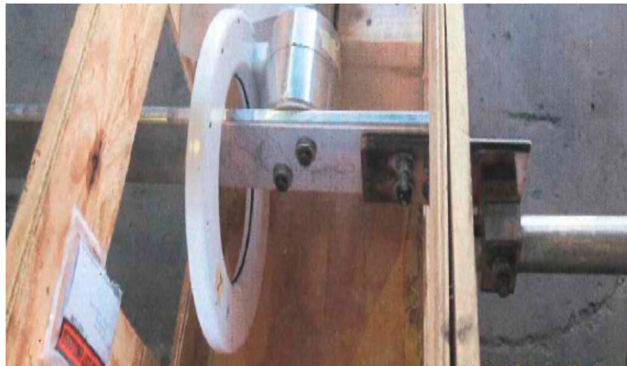
Figure 7. Close-up view of the 132 kV NCIT head with bus bar.
