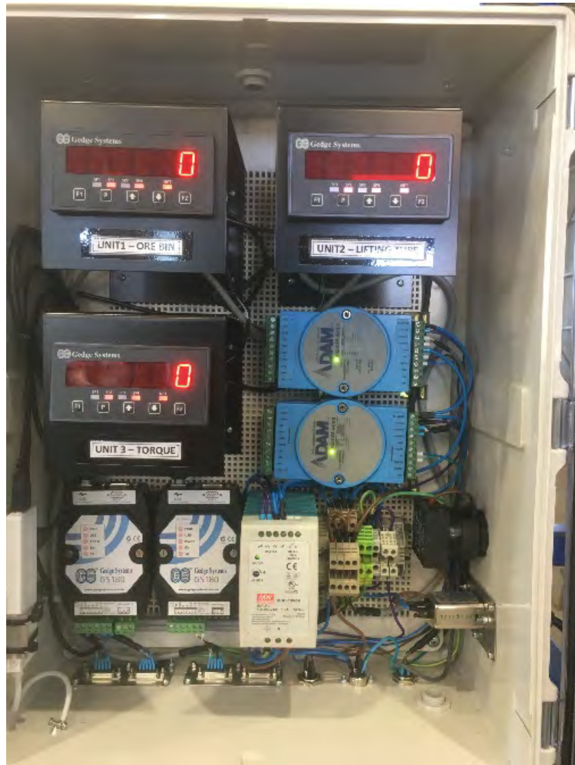
Picture 2E. Test Rig 2 weigh indicators and controllers
