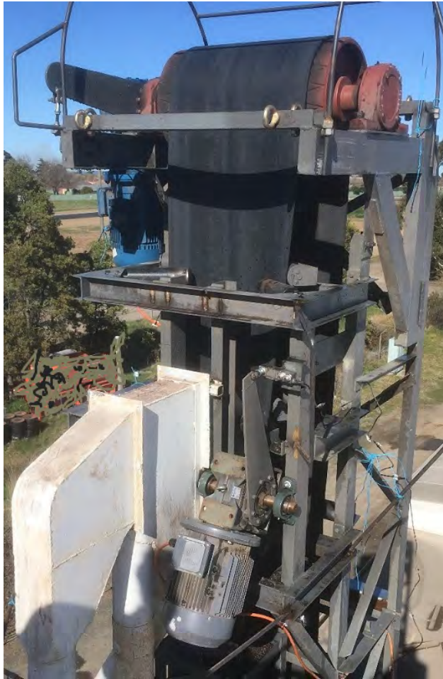
Picture 3D. Top of the hybrid elevator. Showing the load cells of the torque arms for the pipe conveyor and the cable disc elevator
