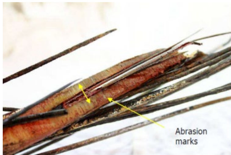
Figure 14: Example of cable break due to abrasion [Ref.16]
