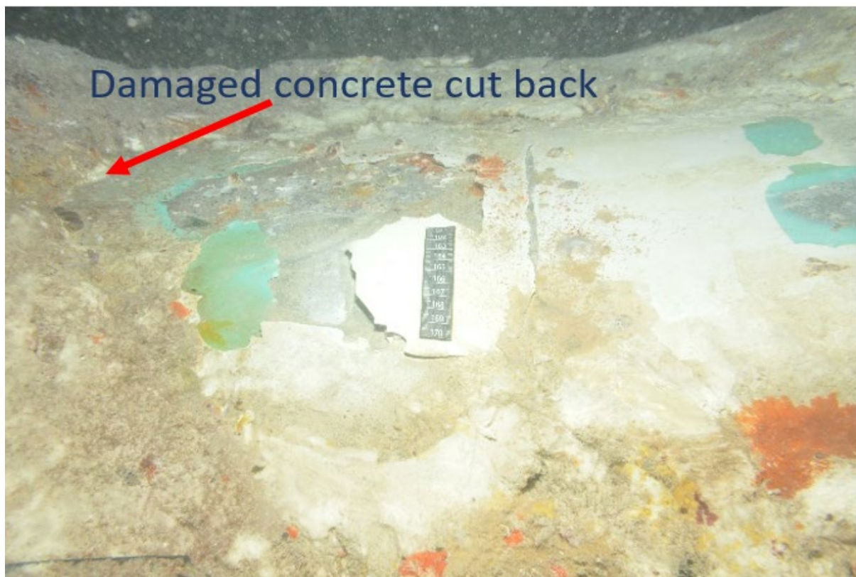
Figure 26: Damaged concrete cut back
