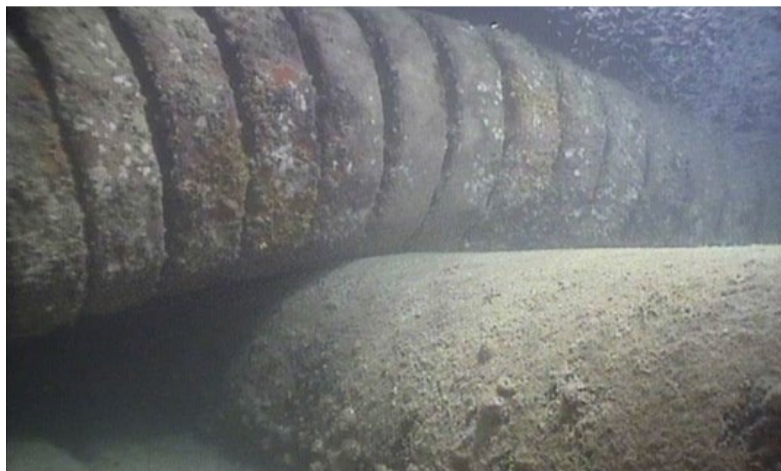
Figure 16: ROV Survey at the crossing locations- Note the articulated padding installed on the crossed pipeline away from the field joint
