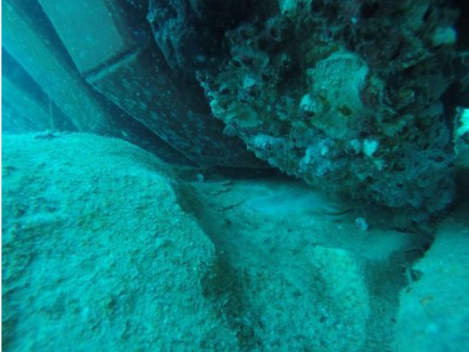
Figure 17: Damaged Field Joint Coating-Pipeline # 1. Note that the cable is not yet lifted for the purposes of inspection in this photograph.
