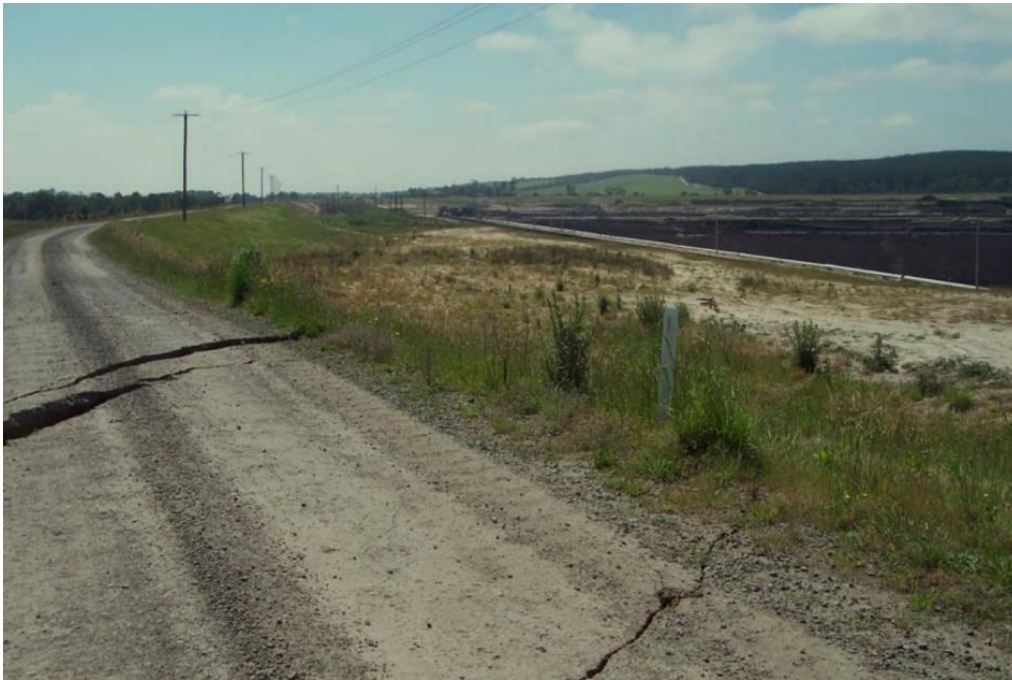
Figure 1.7 Observed cracks on Victorian brown coal batter (Mining Warden, 2008)
