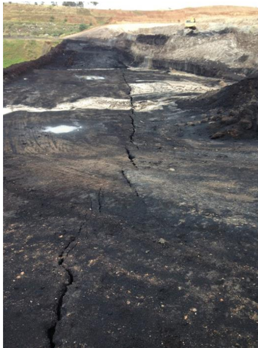
Figure 6.2 Major cracks on north batter in November 2013
