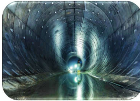
Fig. 3.27: Underground shield tunnel constructed from curved sections that are sealed by compression gaskets. (Photo from the Institution of Civil Engineers.) 209
