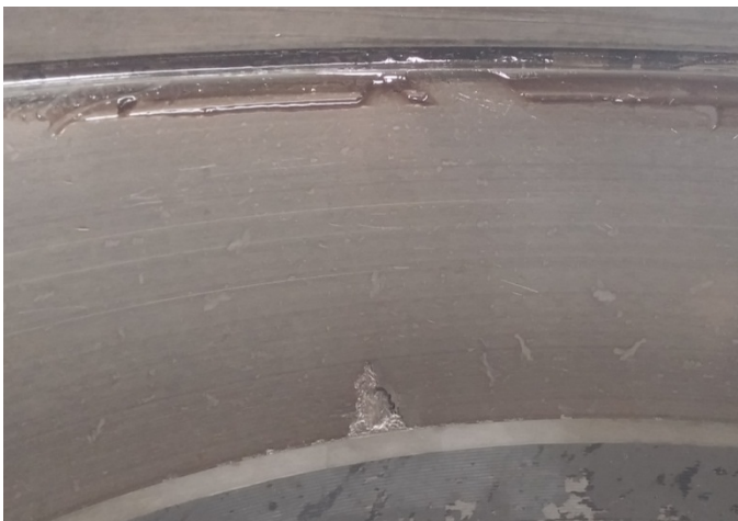
Figure 7: Photograph of a second spall (Spall 2) that developed on the OB raceway of Test Cup A of Bearing 3 after a total of 77,506 miles of operation — 4 th Teardown
