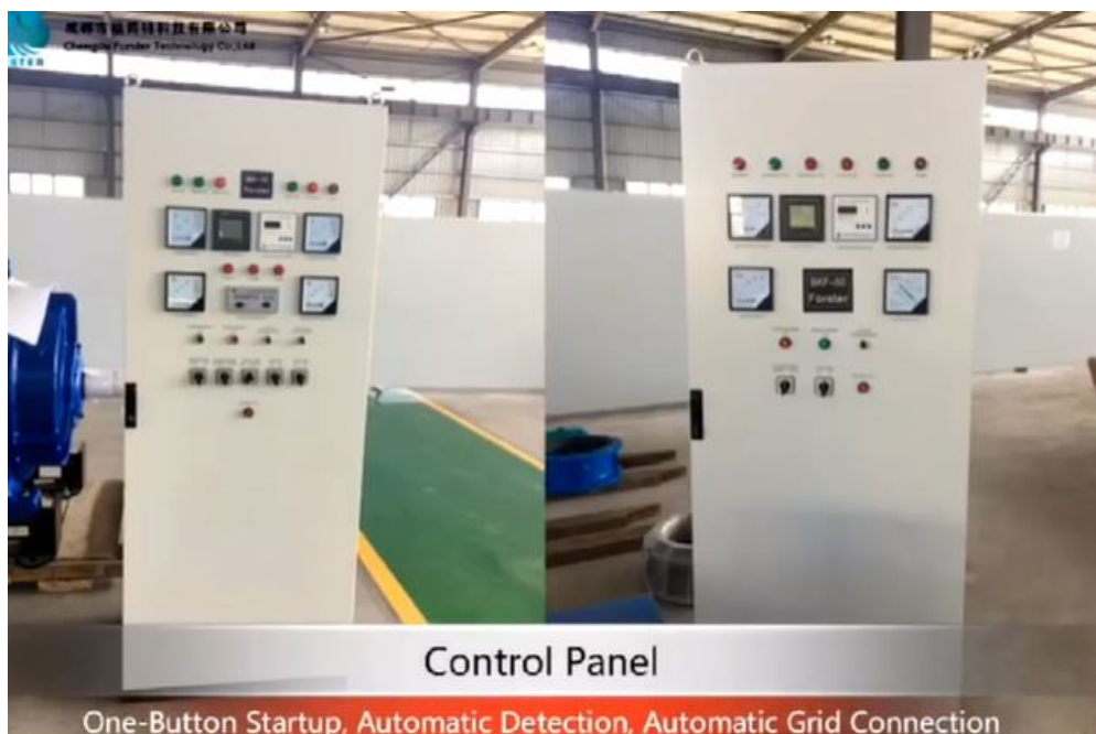
Figura 6. Panel de Control
