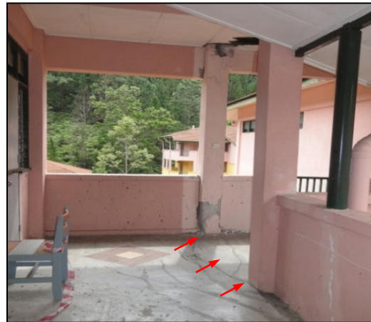
Slab cracks at joint to adjacent building (photo was taken on the 3 rd floor)
