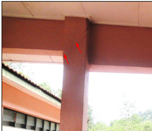
Shear crack at column (photo was taken from the 3 rd floor)
