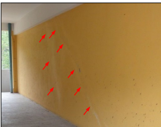
Cracks and sealed brick wall (photo was taken on the 1 st floor)
