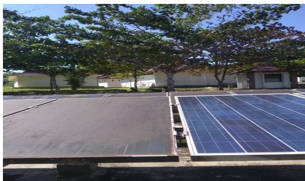
Figure 3. Measurements of photovoltaic before and after cleaning
