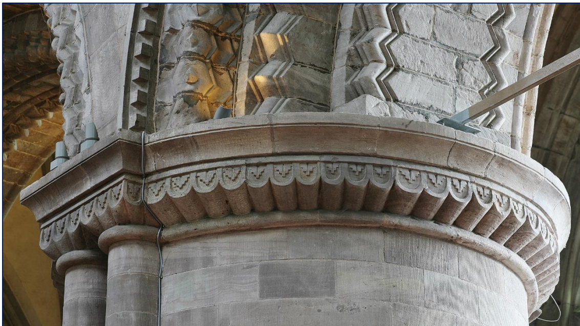
23 Hereford Cathedral, S nave arcade, detail Pier 4, with stepped pattern on the capital scallops in relation to Kempeley chancel arch.
