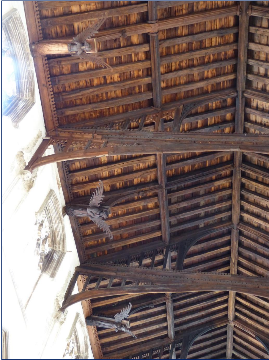
Figure 5 Angel roof, St Nicholas' King's Lynn (Norfolk), 15 th century. Photo: Wikipedia Commons.
