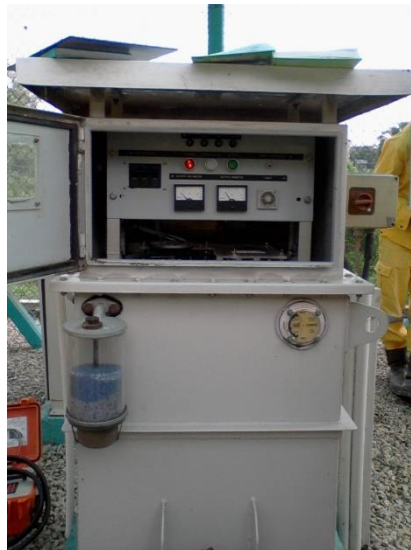
Figure 4: Transformer Rectifier Unit
