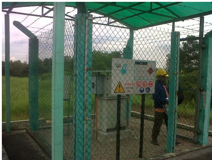
Figure 3: Oil type transformer for cathodic protection station.
