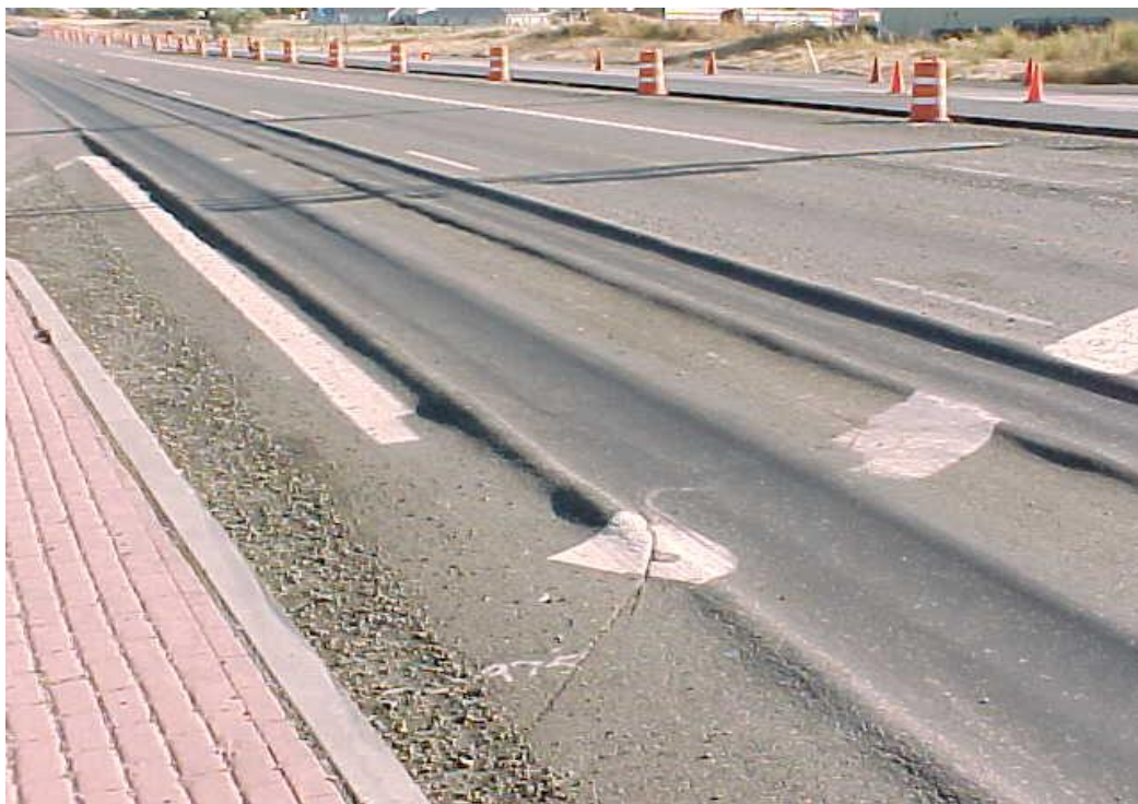
Figure 1.3: Severe ruts in an asphalt pavement
