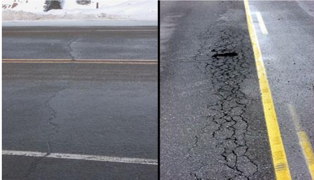
Figure 1.2: Typical longitudinal and transverse cracks
