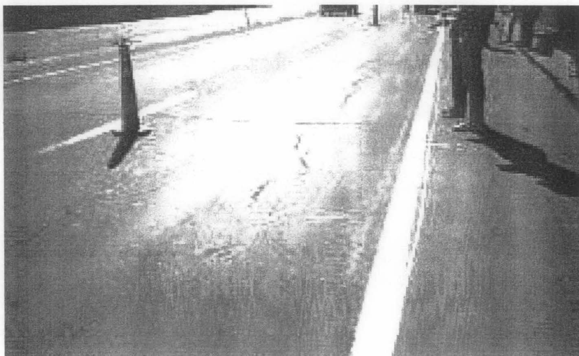
Figure 2.7 Low Severity (Source: FHWA, 2003)
