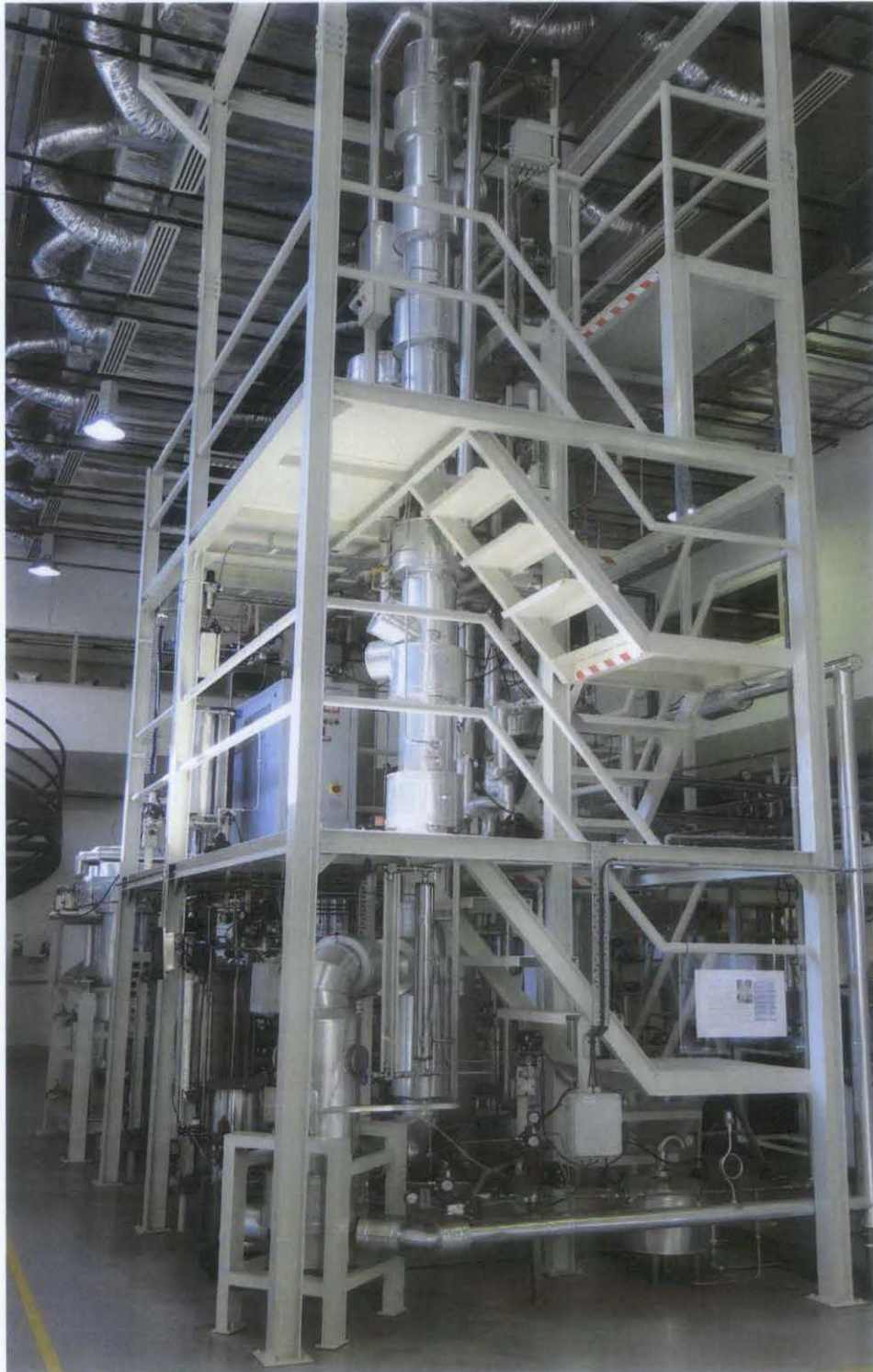
Figure 3.2: Distillation Column Unit.
