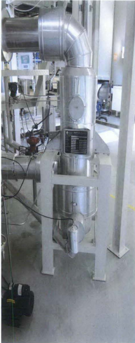
(a) Reboiler Unit
