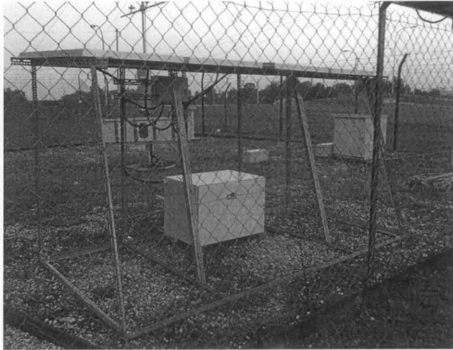
Figure 3.21: Solar Power System installed
