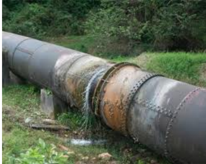
Figure 2.3: Corrosion happen external side of the pipelines
