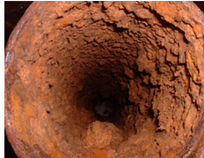
Figure 2.4: Corrosion inside of the pipe
