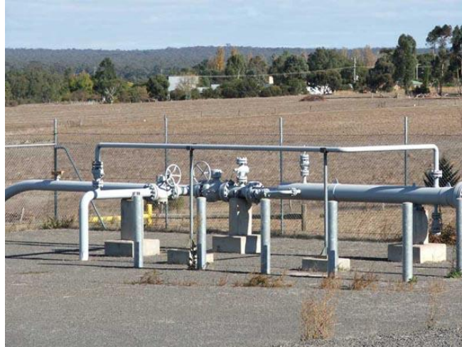
Figure 1: Gas Metering System
