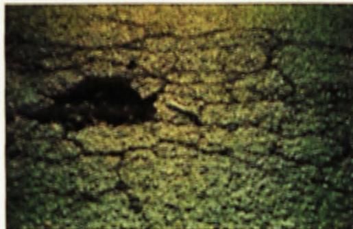
Figure 2.2: Pothole from Fatigue Cracking
