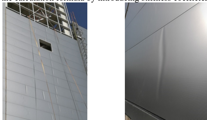
Figure 2. Destruction phenomenon of metal faced sandwich panels under temperature action.
