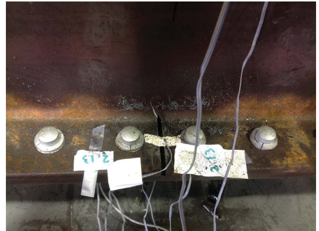
Figure 11: Artificially induced fatigue crack propagating into the web for new equivalent girder.
