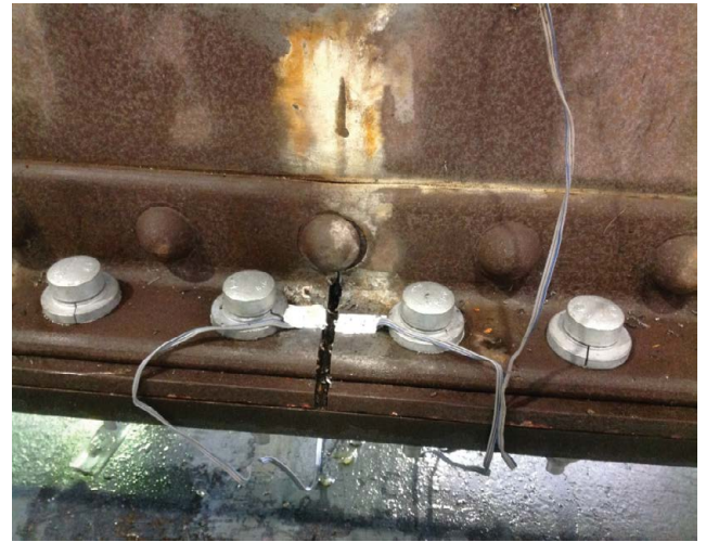
Figure 16: Artificially induced fatigue crack propagating into web of RMS 120-year-old-girder.
