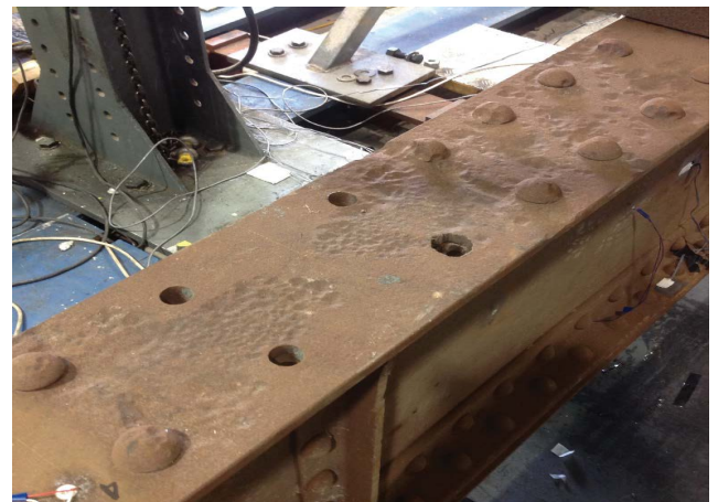
Figure 4: Defects for 120-year-old girder.
