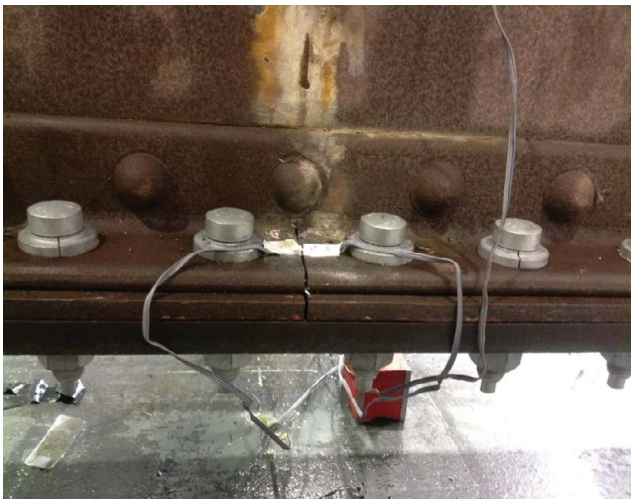
Figure 15: Artificially induced fatigue crack for RMS 120-year-old girder.
