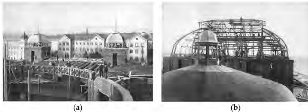
Figure 1. (a,b) Views of the National Theater of Zagreb during its construction. Provision courtesy from Hrvatsko Narodno Katalište u Zagrebu.
