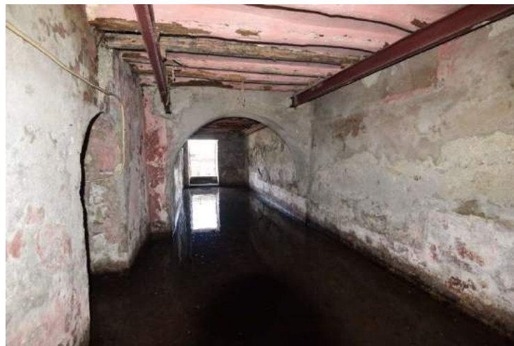
Figure A11. Flooded ground floor in a building along the coast of Marina Lunga. Until the 1980s, it was used as warehouse, but later, it was abandoned due to sea level rise. Presently, the ground floor is below the local sea level.
