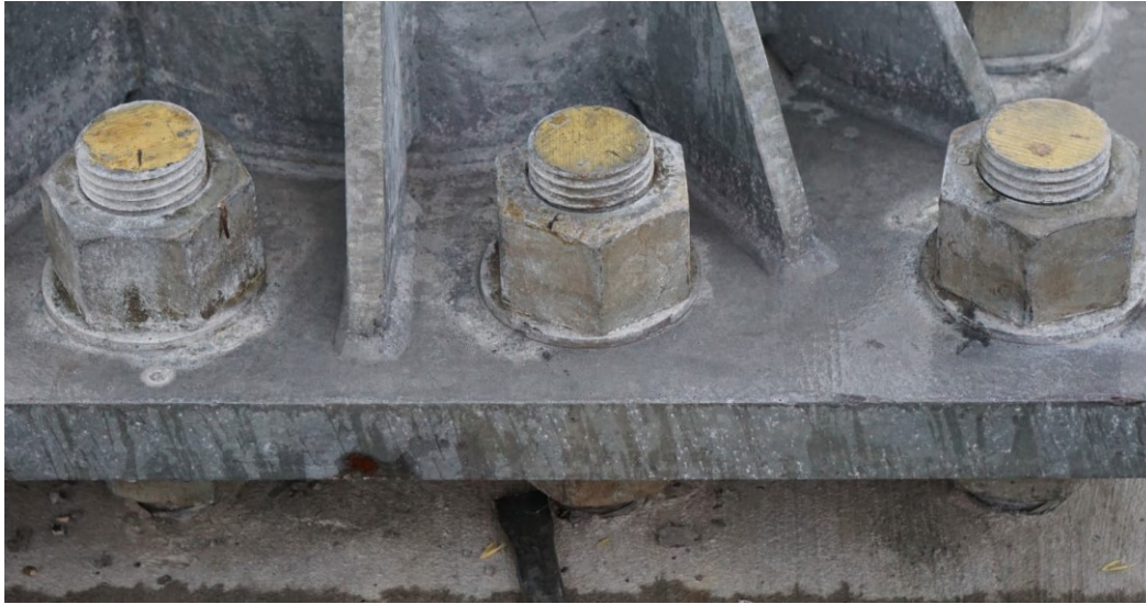
Figure 2.3. Rod 8 out of plumb
