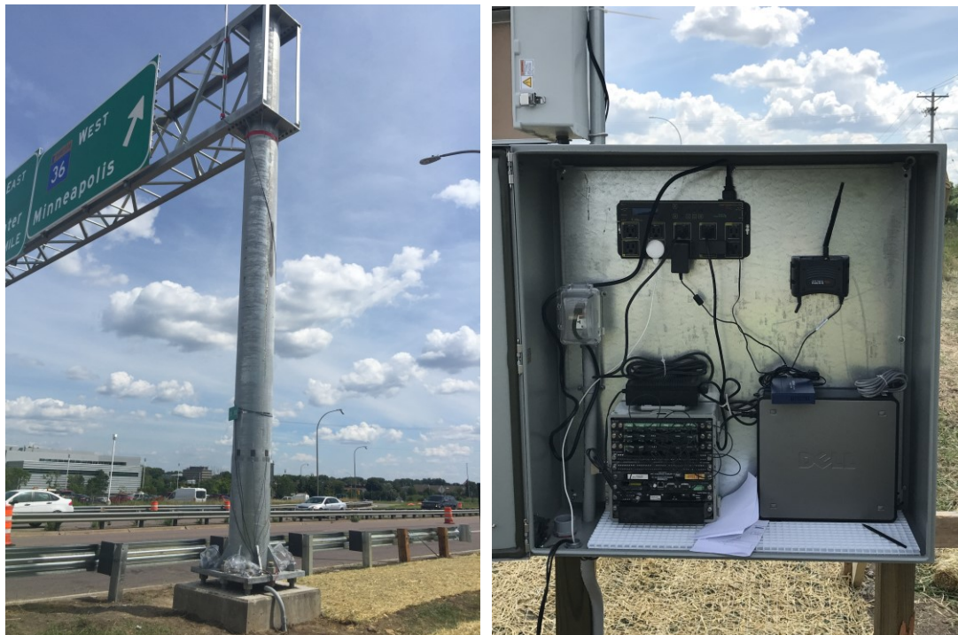
Figure 5.1. Instrumented sign post (left) and data logger cabinet (right)
