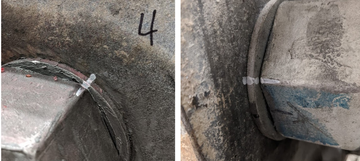
Figure 3.4. Turn marks after tightening on top (left) and on leveling nuts (right)
