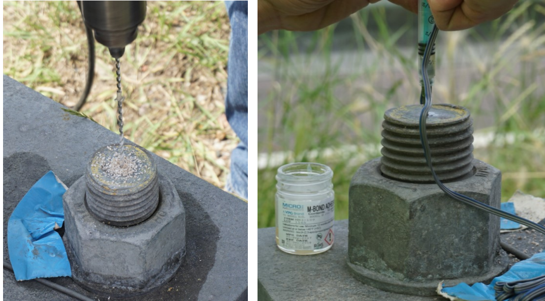
Figure 5.4. Drilling out failed strain gauge (left) and replacing strain gauge and injecting epoxy (right)
