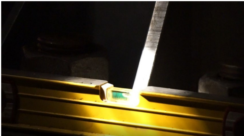
Figure 2.4. Final installation of OH 280-023 out of level
