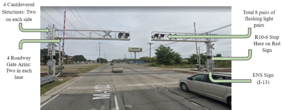
Figure 8: Existing Warning Devices for 8-Mile Road
