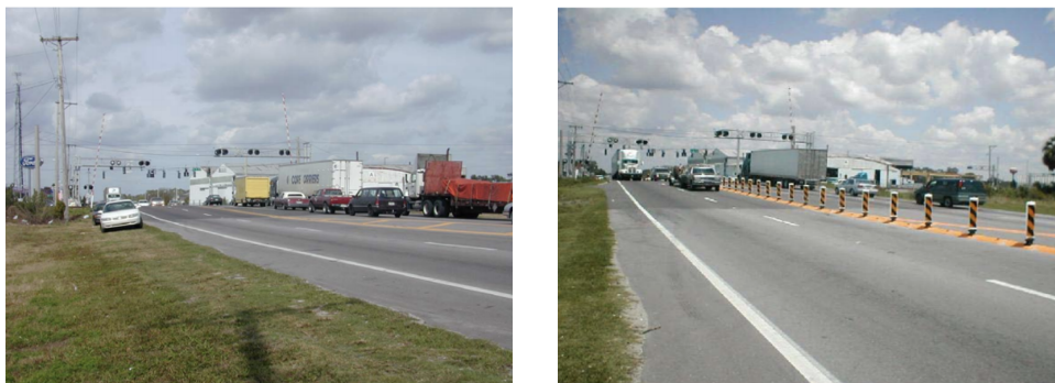
Figure 29: An Installation of traffic channelizers at a crossing. Source: (Ko, Courage, & Wilis 2003)
