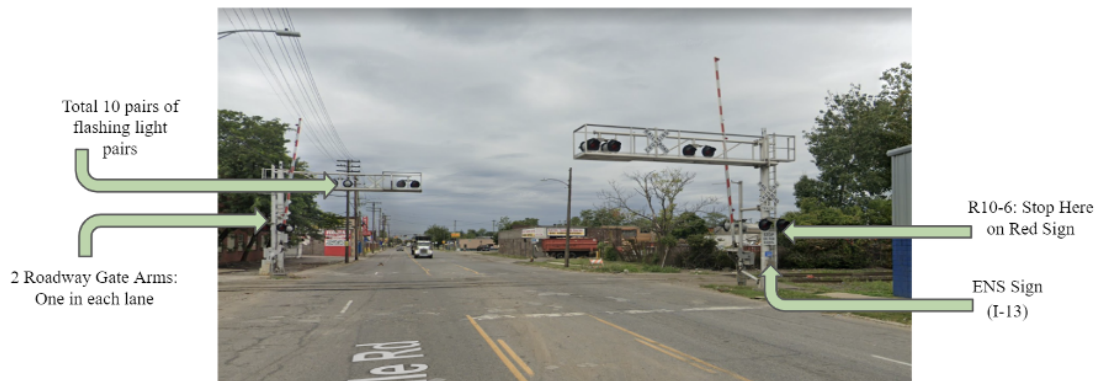
Figure 5: Existing Warning Devices for 6-Mile Road
