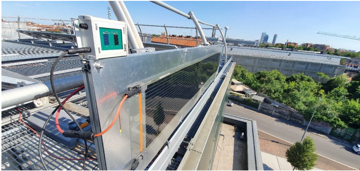
Figure 4. OPV module facing west (OPV-W) installed at the edge of the test facility.
