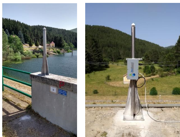
Figure 2. Steel pillars supporting the antennas for points PT3 (left) and PT4 (right). The other points are materialized with the same kinds of structures.
