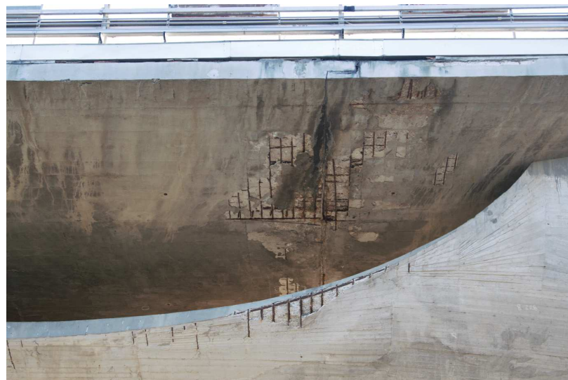
Figure 7. Deterioration of Gerber saddles and underlying vault.
