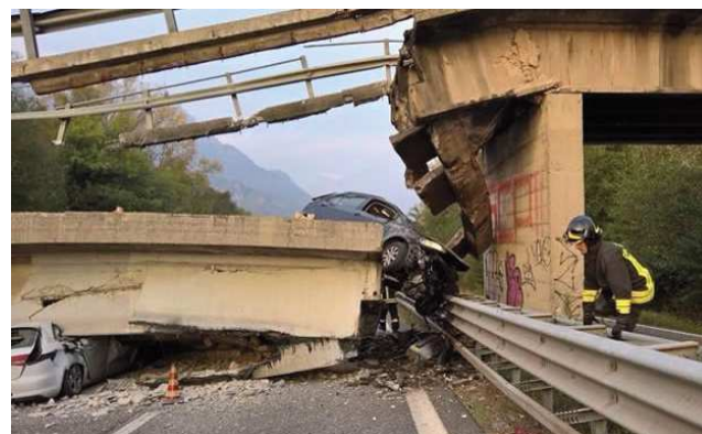
Figure 2. The Annone Brianza overpass collapse.
