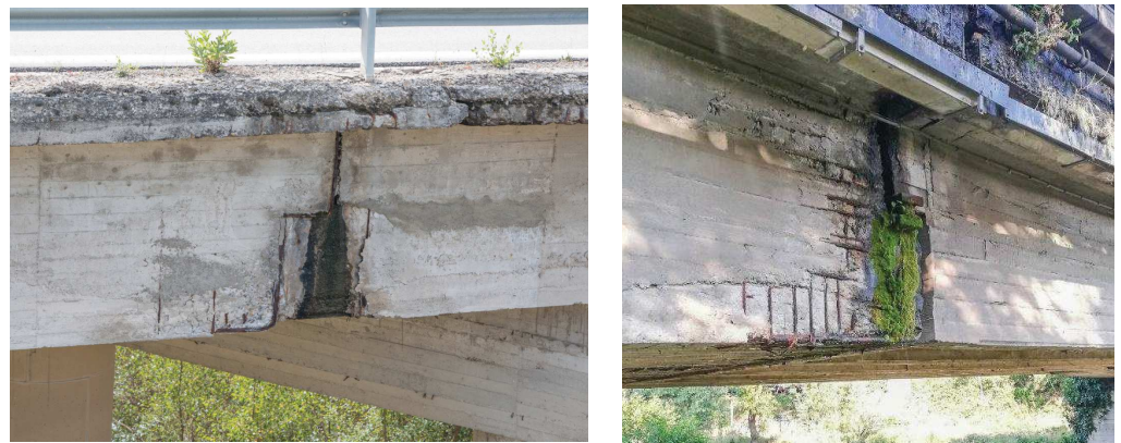
Figure 1. Examples of deteriorated Gerber saddles in RC road bridges.
