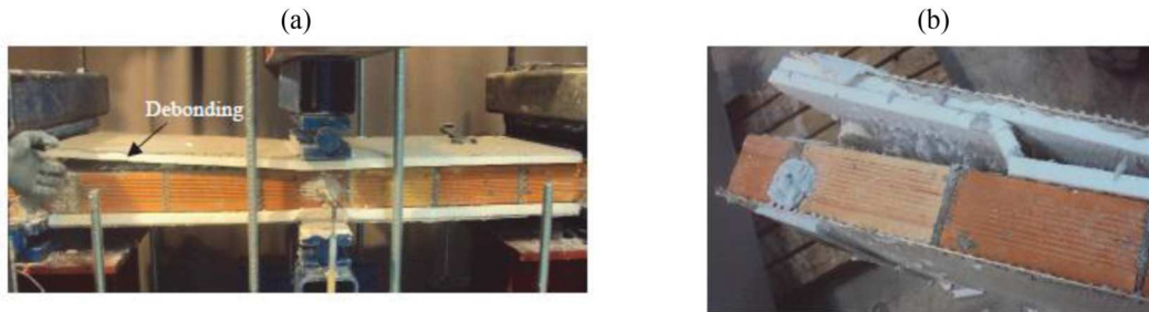
Fig. 11. Debonding at the insulation-masonry interface (a) one layer; (b) two layers of insulation [64] - CC BY 4.0).
