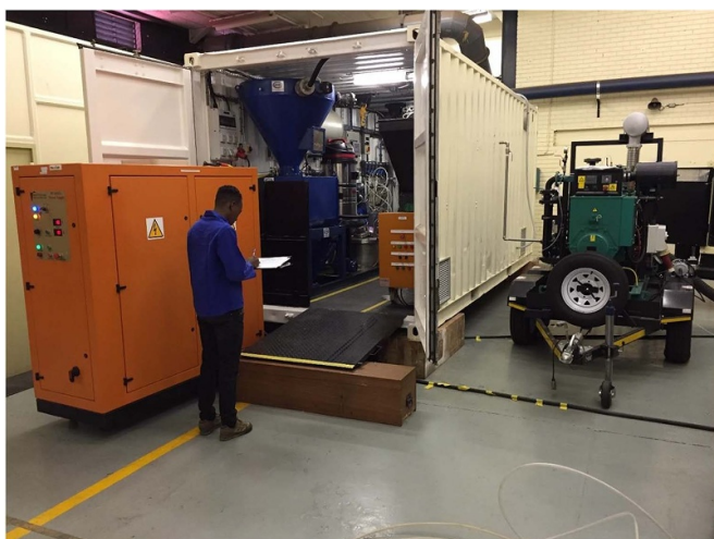
Figure 29. Containerized plasma waste to energy system.
