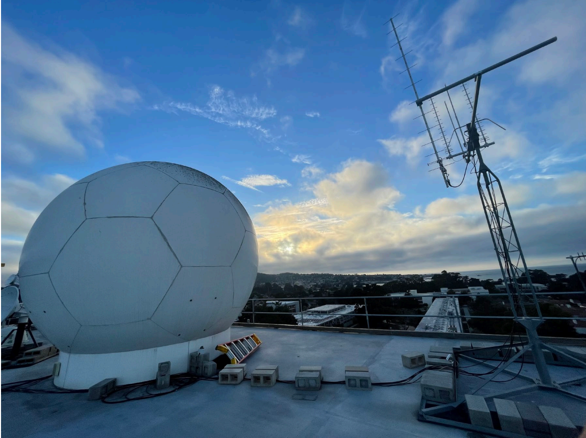
Figure 12. UHF Yagi and S-Band 3m dish dome. Source: NPS (2022).
