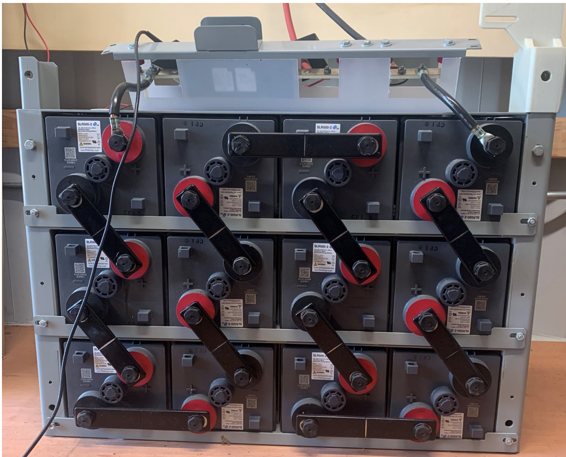
Figure 3.8. The batteries used in the microgrid setup include 12 2-V lead-acid (primary compound) batteries in series.
