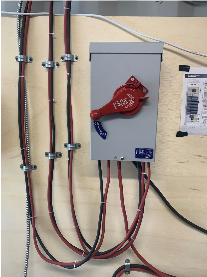
Figure 3.4. The three strings of four solar panels in series are combined into one power source through the combiner box.
