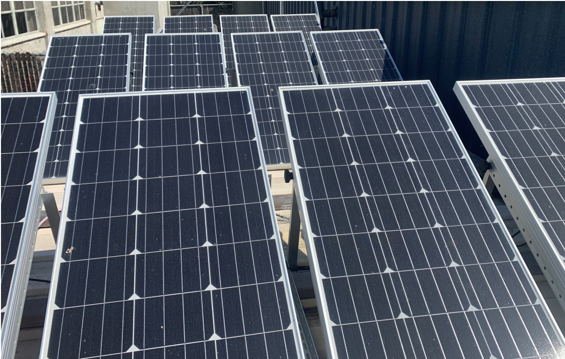
Figure 3.3. The 12 solar panels used at this microgrid provide 1.2 kW of power.
