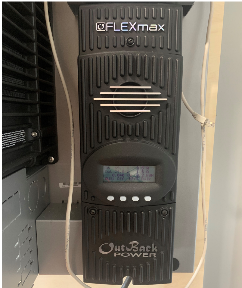
Figure 3.5. The charge controller's primary goal is to maximize the incoming solar power and convert it to a nominal level for the batteries.
