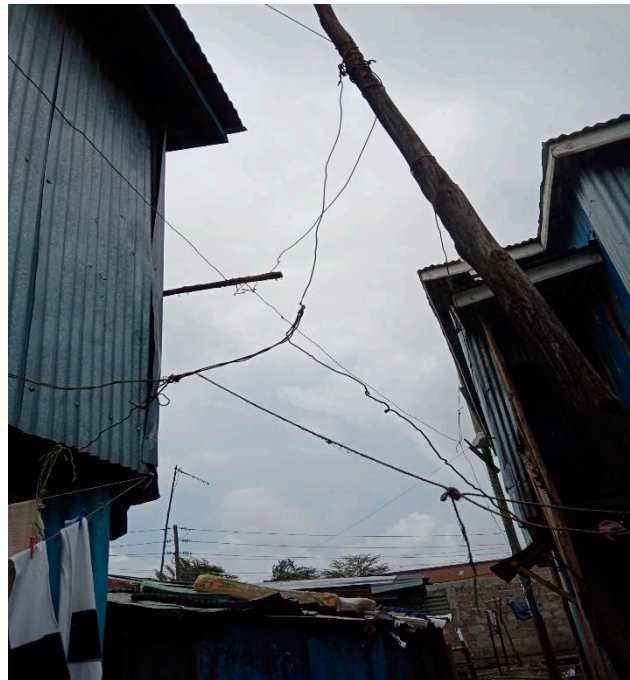
Figure 1. “So, the [electricity] wires are actually stima za kusambaza (illegal electricity connections), they are very dangerous. They can electrocute when wet . . . at night you cannot sleep because they start producing sparks . . . there is a time they burnt a house” (Daniel, 17-year-old boy, Viwandani).
