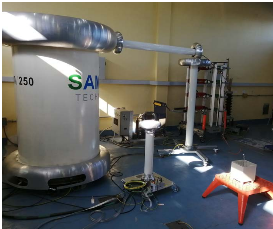
Figure 6.4. Step up transformer and test cell for the AC BDV tests
