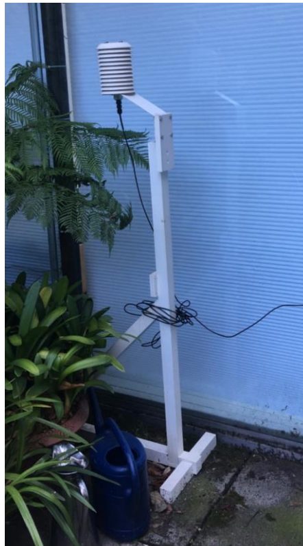
Figure 43: External dry-bulb air temperature sensor
