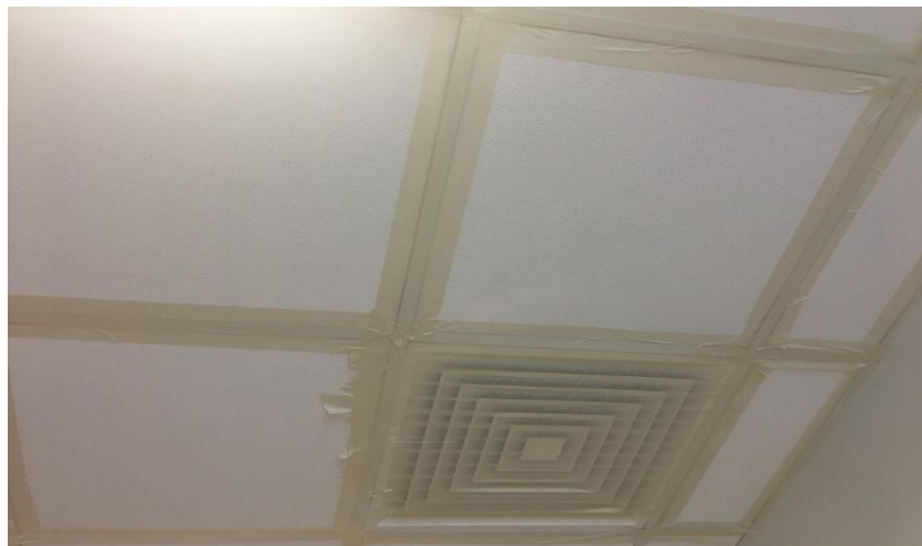
Figure 49: Application of insulation of the ceiling diffusers and edges around the ceiling tiles.
