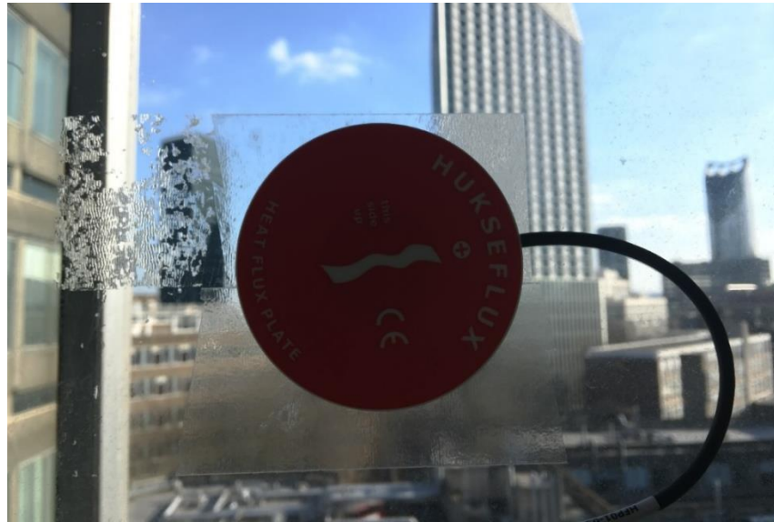
Figure 57: HFP01 Heat Flux sensors mounted on the internal central part of the glass with a double-sided TESA 4939 tape.
