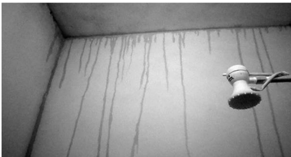
Figure 17 Water Damage In The Toilet Of A House In The Resettlement (Photo By MAB 2014)
