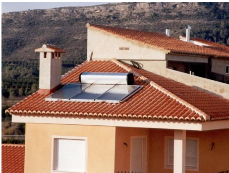
Figure 26a. Type a) Domestic Solar Hot Water System on the roof of a building (Photo: Solahart/ESTIF 2016)
