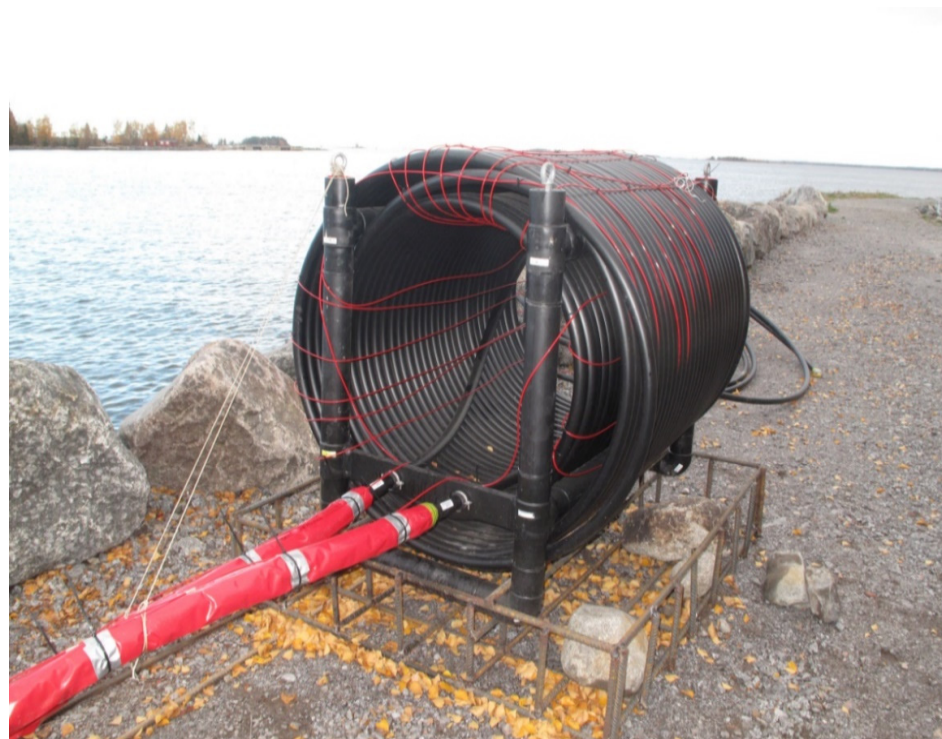
Figure 3. The water heat exchanger that was planned to be installed in Merten Talo is connected to the tubes (of the heat pump in the home), which are insulated. The red wire is the temperature sensors (Picture taken by Anne Mäkiranta during installation process 18 October 2018).
