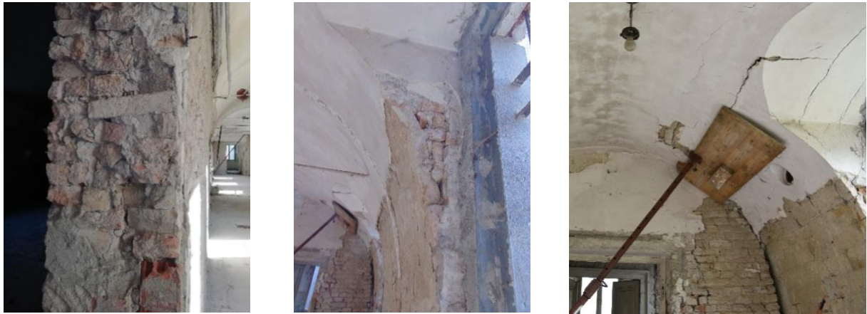
Fig. 3: On the left the masonry of poor build quality. The center photo show the bad construction quality of the vault. On the Right the the north-eastern corner with the collapse of the vault which has led to the insertion of a temporary prop.
