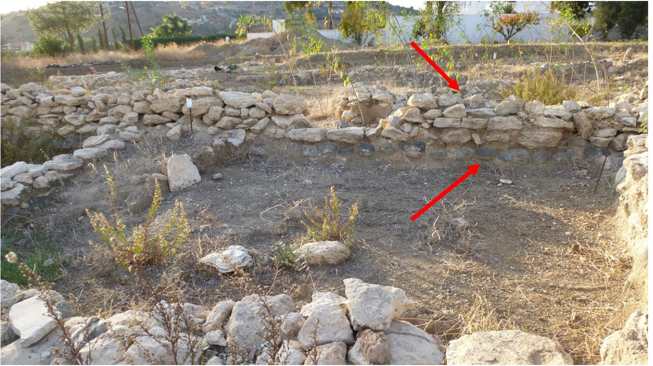
Figure 3.4 Pyrgos foundations with limestone levels overlaying on a double level of basalt blocks (picture by the author).
