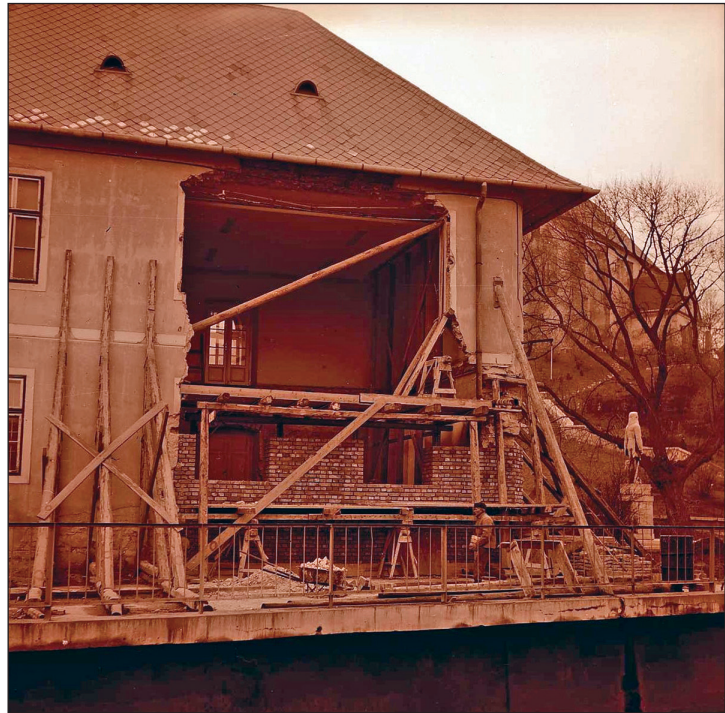
• Fig. 4. • The damage of the museum in 1967. The collapsed northern façade after the disaster (Photo by Levente Szepesi Szűcs, 1967, HOM FN 19178)
