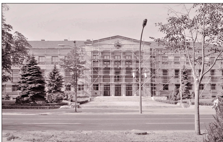
• Fig. 10. • Reconstruction for museum purposes finished in 1980 (Photo by Ede Valent, 1980, HOM FN 47307)
