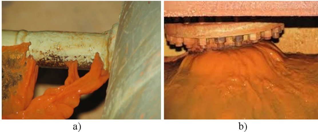
Figure 1: Photos of the accident with the spill of radioactive decontamination solution at the Ignalina NPP (Lithuania, 2010): view of the broken pipeline (a), general view of the spill part (b) [34].
