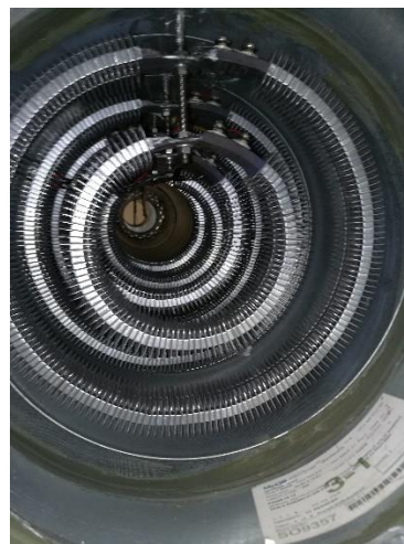
Figure 3-5: Four Sets of heaters
