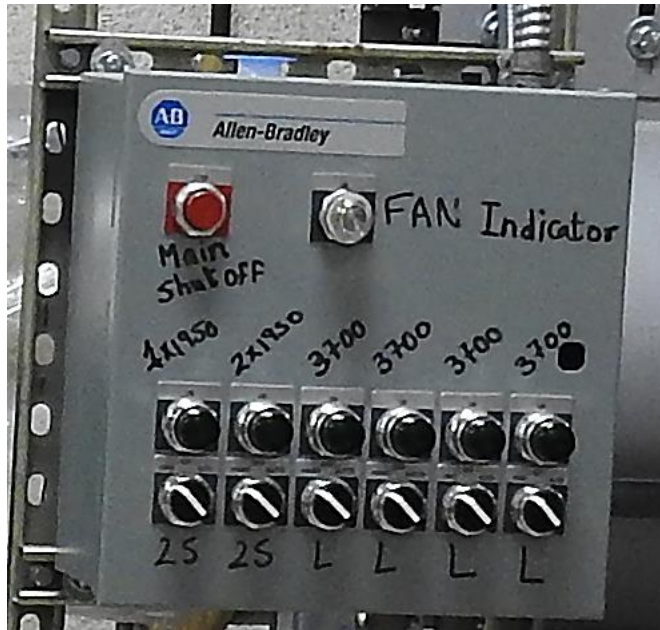
Figure 3-4: Control panel for all the heaters.
