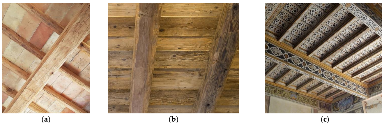
Figure 1. (a) Tiles, rafters, and beams; (b) timber beams and boards; (c) decorated timber beam floor: tiles, and two layers of rafters and beams.
