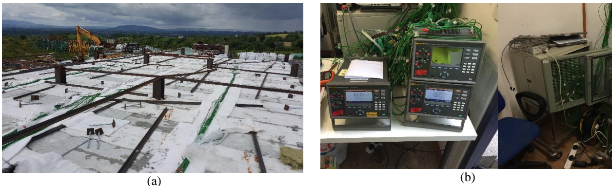
Figure 4: (a) Extension cables used for data recording purposes, (b) Multiple data loggers used
