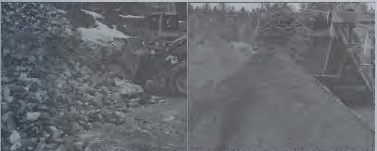
At left, the loader scoops piles of recycled glass and pours it onto the bed of the crusher, which reduces the glass to the fines shown at the right.
