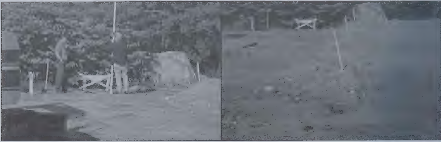
Above left, Bob Harrington (highway foreman) and Bob Ells (foreman from Trumbull-Nelson) set grade stake. At their right and in the right-hand photo, the glass-gravel mix is used to bring the ground up to grade.
