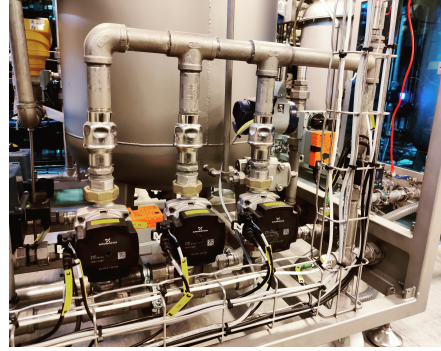
Figure 6: Example of a pumping station module with three pumps in parallel at the SWIL.
