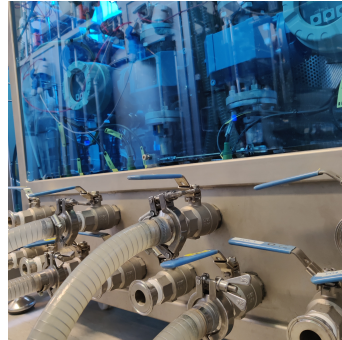
Figure 8: Example of a pipe module at the SWIL with inlet valves, folded pipelines and sensors.
