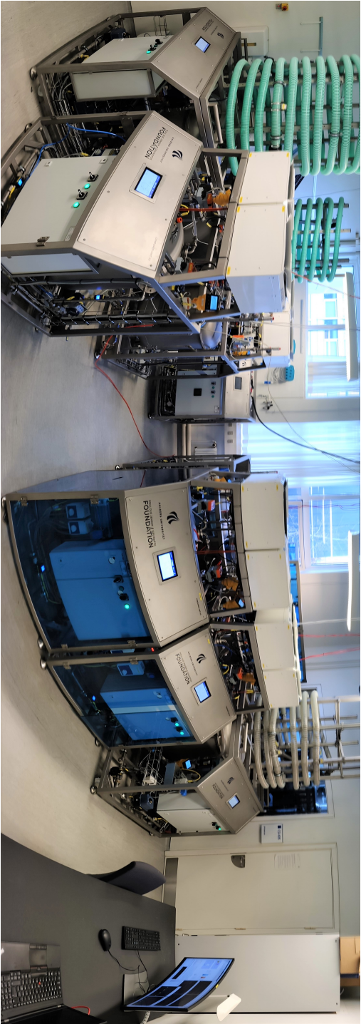
Figure E.1: Picture of the SWIL with two test-beds and the SCADA-PC: (Left) Waste water collection. (Center) Water distribution network. (Right) SCADA-PC.
