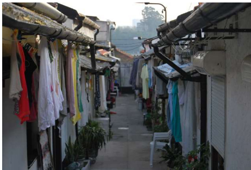
Figure 4: “Ilhas”, the housing typology that the programme will be focused on (source: A. Varea)
